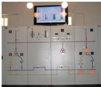
Figure 1 – High voltage substation control shield with additional monitor
